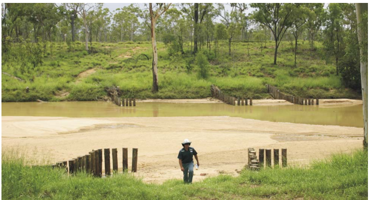
Environmental Graduate, Tom Hayes, inspecting a section of the Isaac River subsidence stabilisation works after rain and associated river flows.
