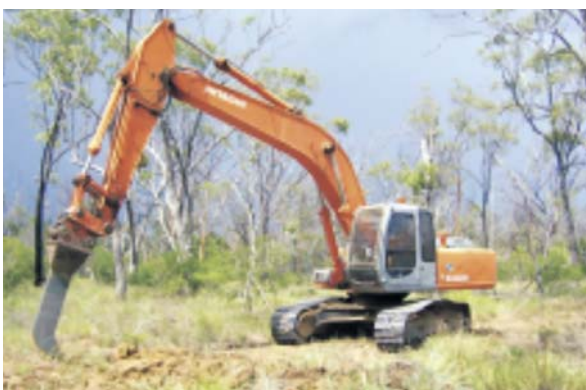
A 24-tonne excavator with the attachment that was developed specifically for Moranbah North Mine subsidence rehabilitation.
