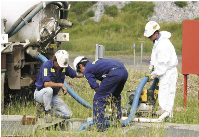
Contractors (from left) George Thrift and Daniel Wisemantel assist Paul Tierney in removing waste sludge from workshop drains and washpad sumps.
