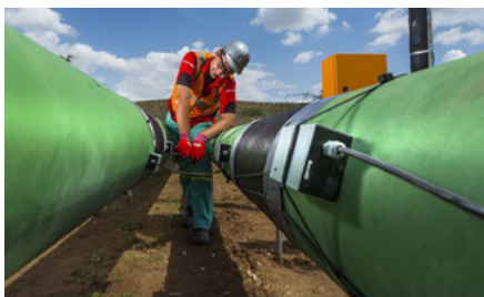
Inspection of fibre optic flow meter installation at Mogalakwena PGMs mine, South Africa.
